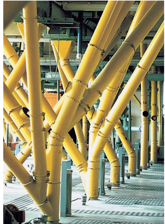
▲ Piping and distribution systems acc. to the modular component system for bulk-product handling as well as for ventilation systems in pressure surge resistant design up to 3 bar overpressure, in standard steel and stainless steel execution
